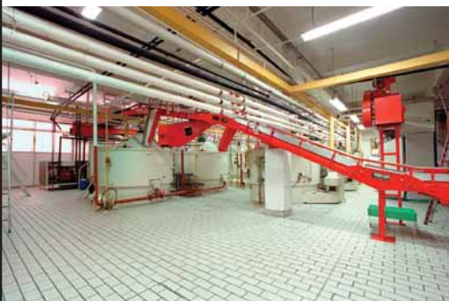
HACCP-compliant production facilities, ION Faliro
